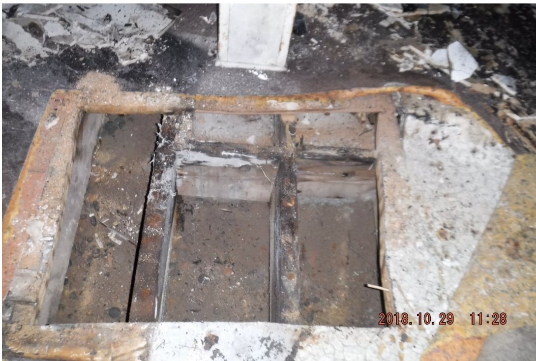
Photo 10 - Water Damaged Floor Joist Area M2
