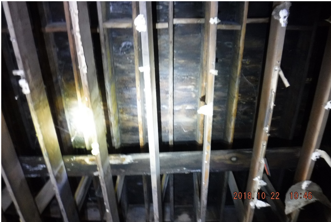
Photo 17 - Ceiling & Roof Water Damage Area S1
