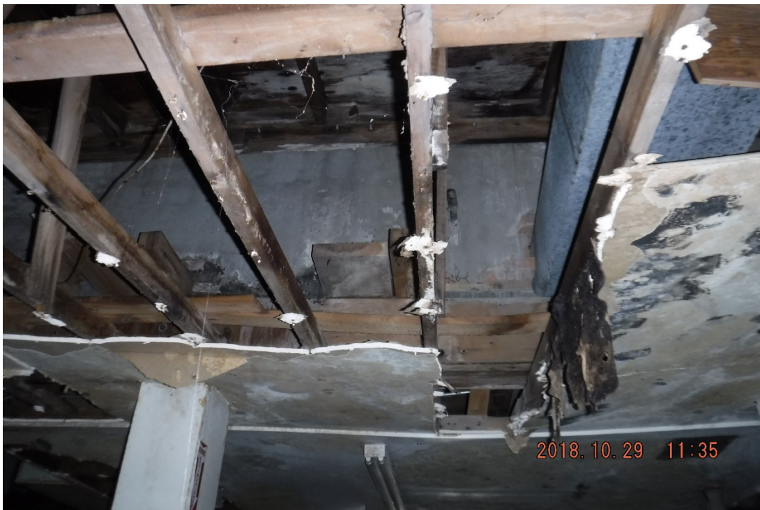
Photo 12 - Damaged Support Below Masonry Wall Above Gridline C
