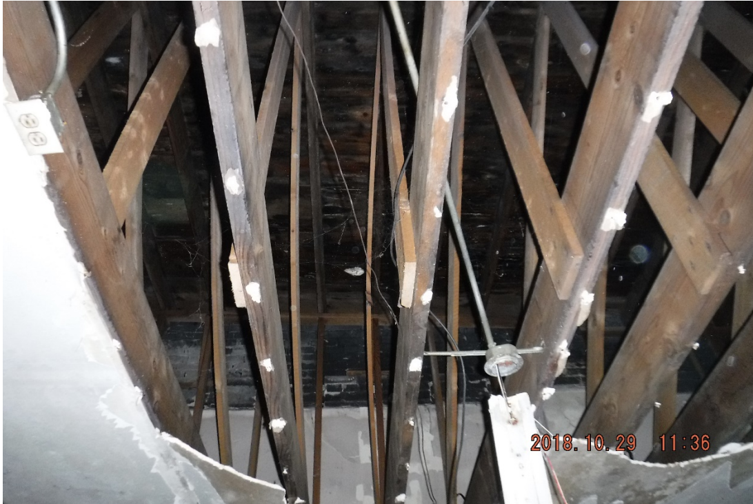
Photo 5 - Truss Bowing Area M1
