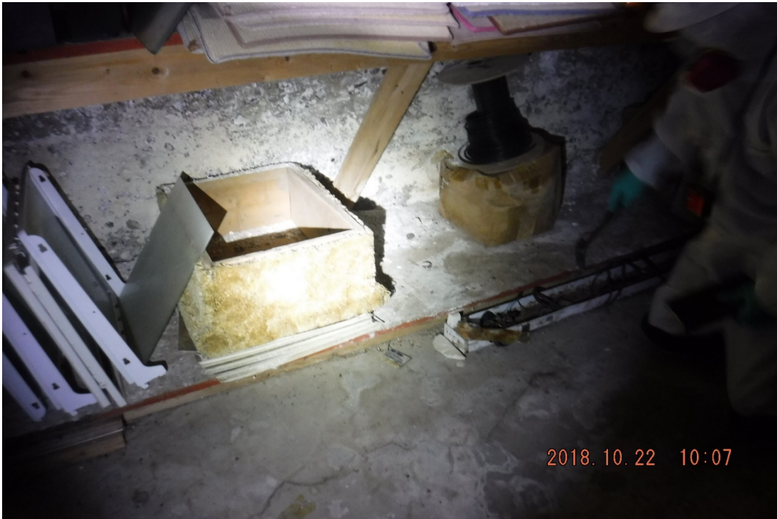
Photo 4 - Basement Wall Deterioration
