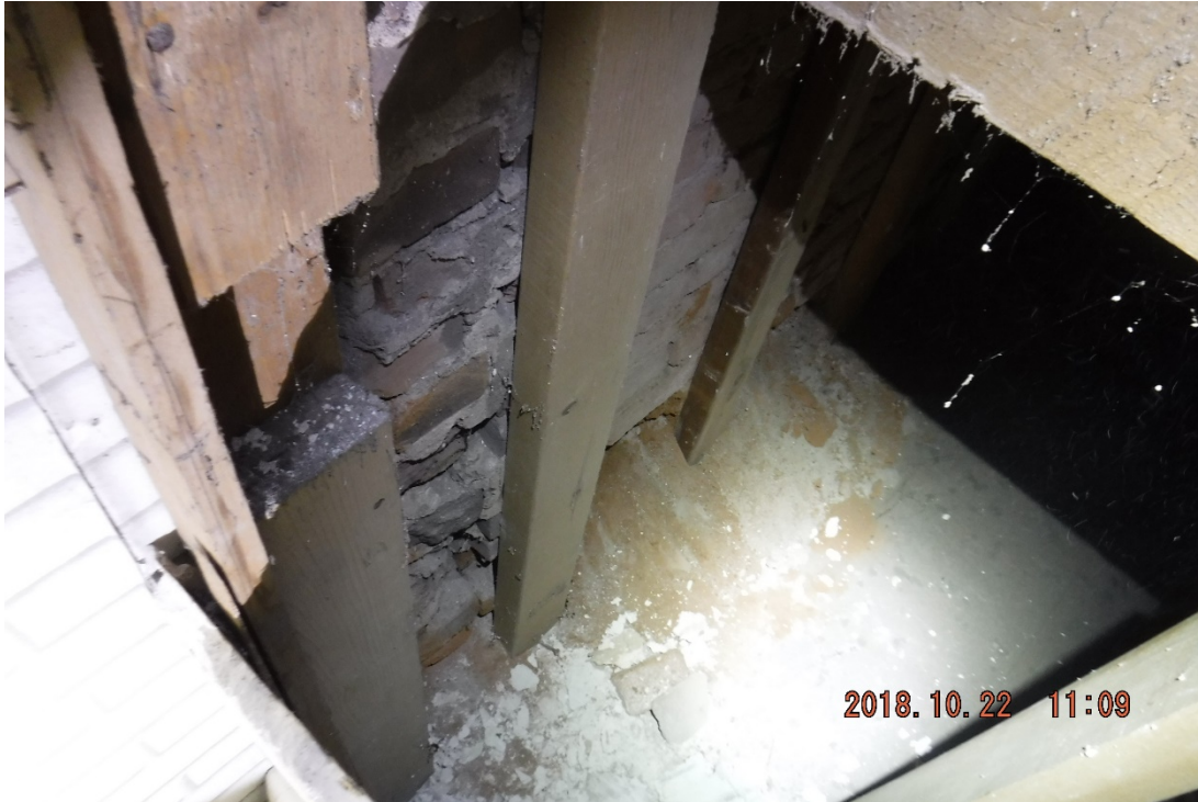
Photo 13 - Deteriorating Masonry At Gridline C
