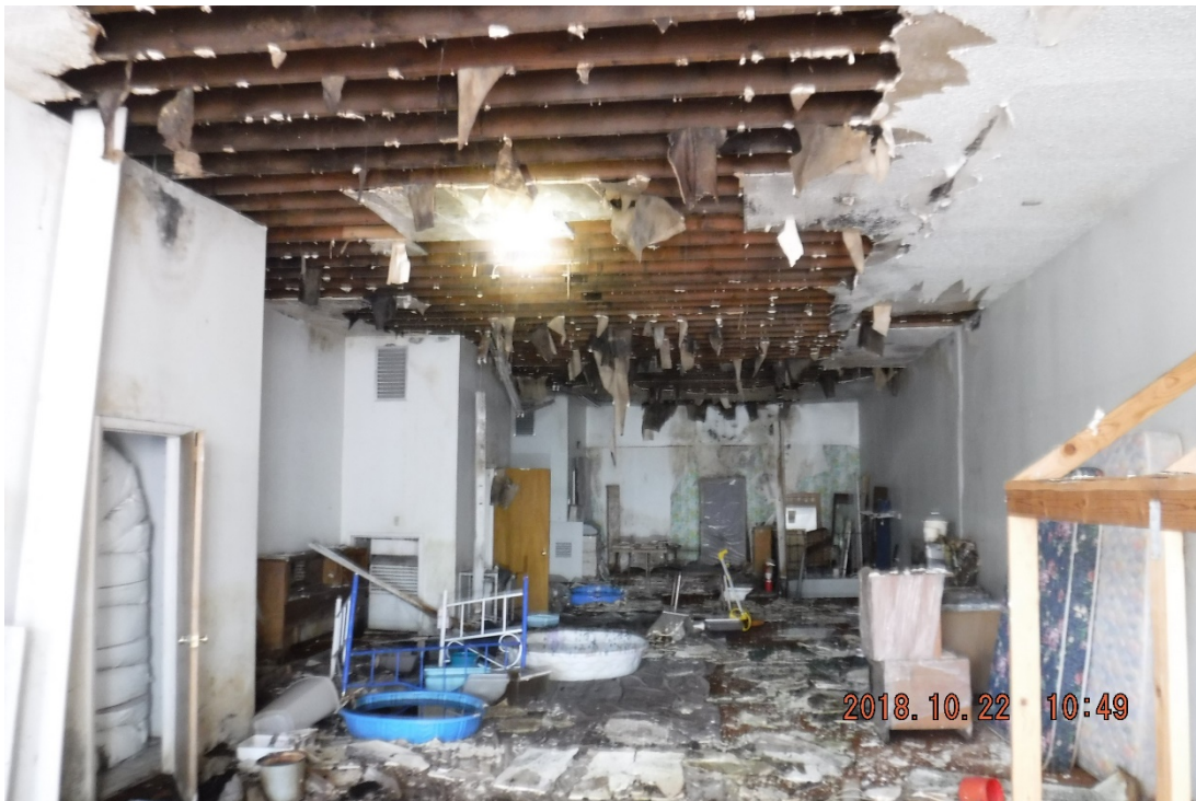
Photo 14 - Water Damage Area S1
