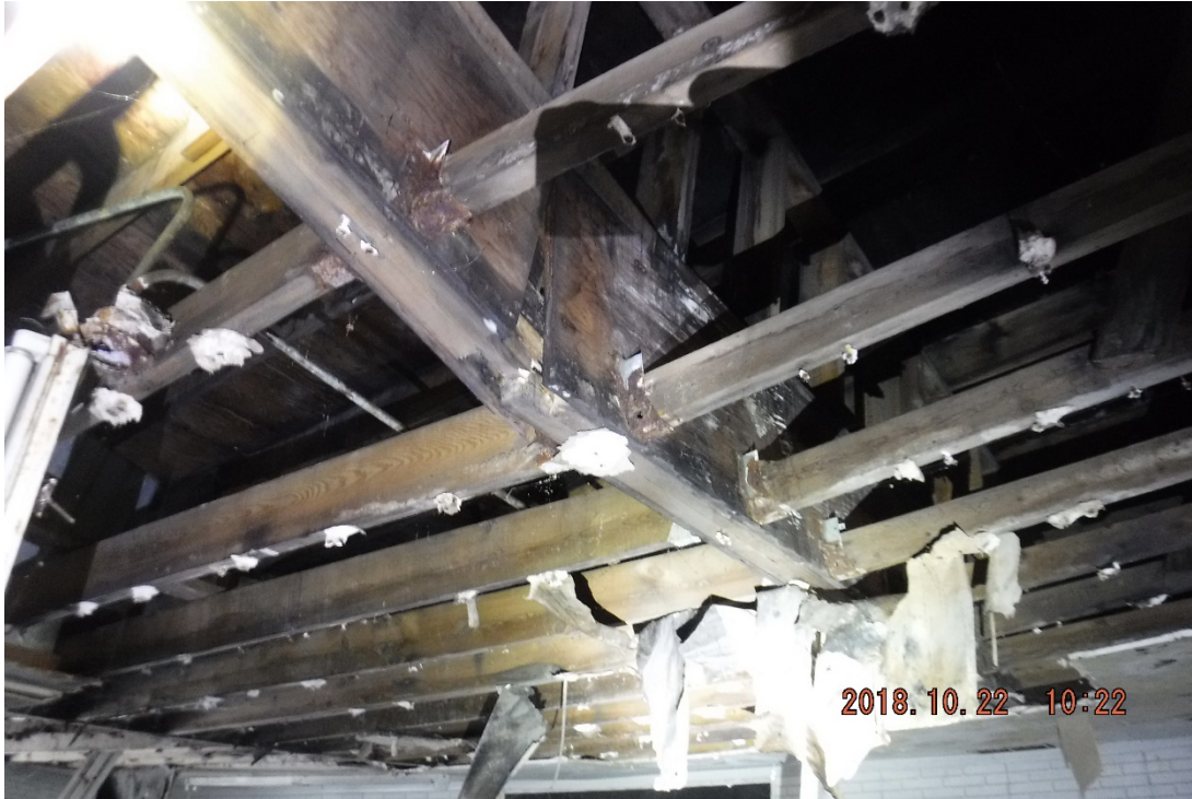
Photo 11 - Broken Structural Member Area M3
